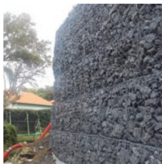
Bulging of the front face
