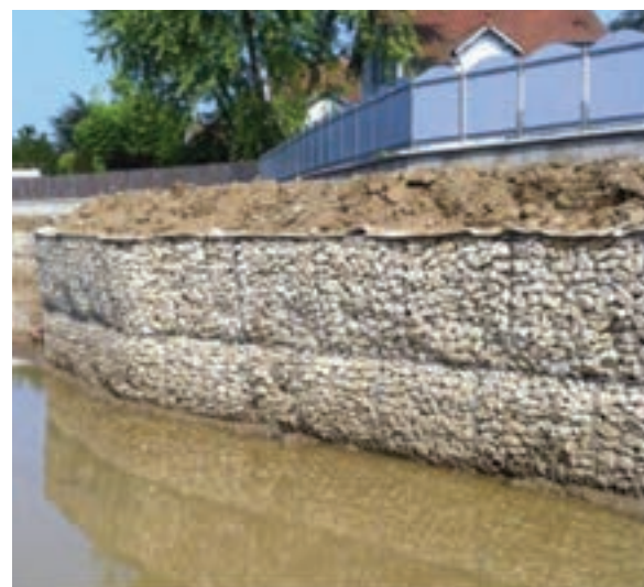
Settlements and distortions of the structure
