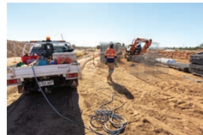
Fig. 3 - Compressor mounted in the tray for mobile use
