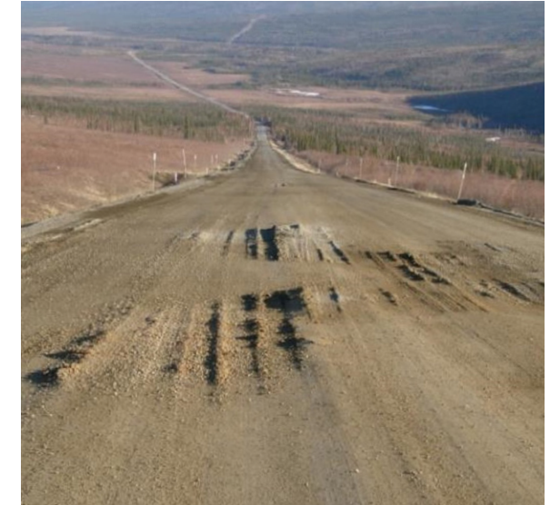
Basecourse rutting due to thaw weakened subgrade
