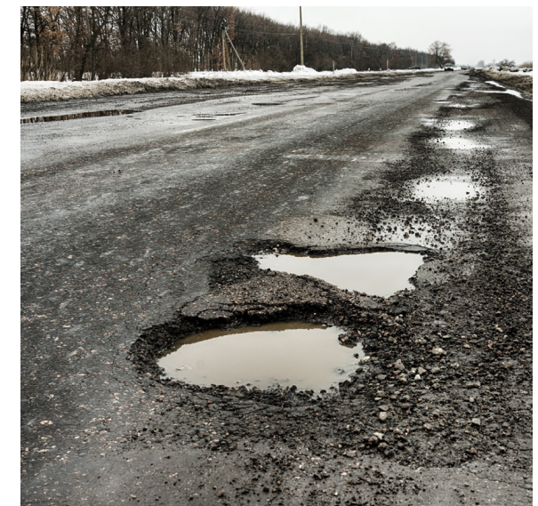
Frost boil through cracked pavement surface
