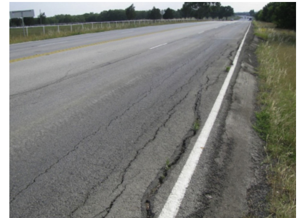
Longitudinal pavement edge cracks in road over expansive clay subgrade
