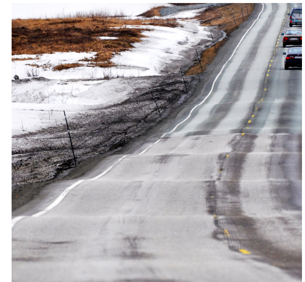
Pavement surface heave due to frost action in subgrade
